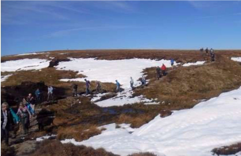
Newly paved footpath as part of the blanket bog restoration on Hartley Fell, Cumbria
